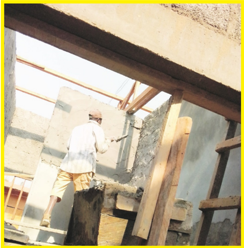
Figure2: Views of the unfinished Lafe Baleng/Bafoussam isolation centre at the time of the on-the-spot control on 29 January 2021
