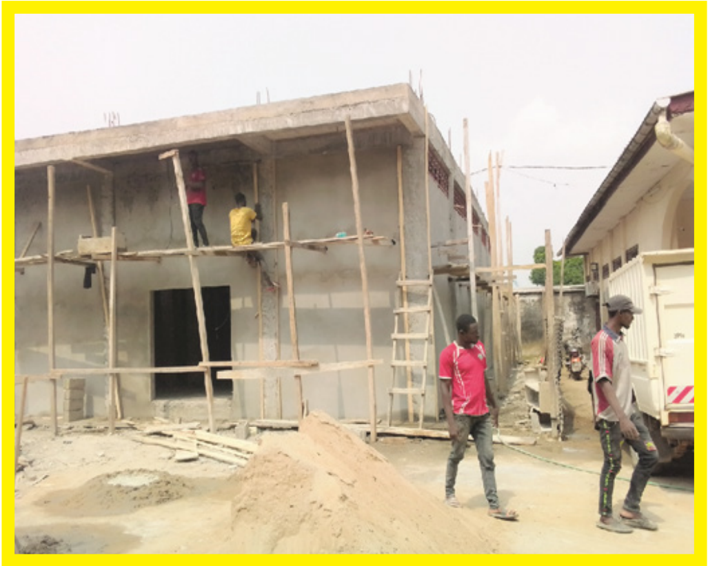
Figure3: A view of the warehouse for inputs and other pharmaceutical products at the Regional Funds for the Promotion of Health in Littoral/Douala, unfinished at the time of the on-the-spot control on 25 January 2021
