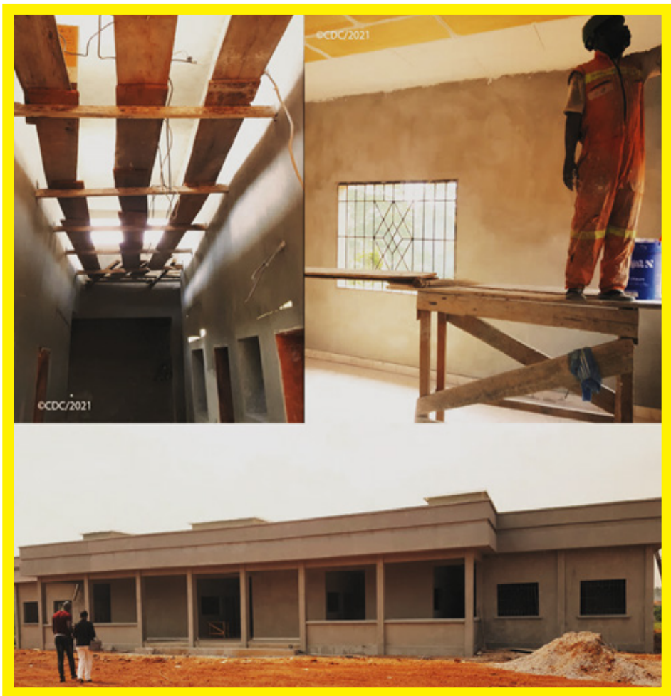
Figure 4: Views of the border health post at Yaoundé-Nsimalen International Airport, unfinished during the on-the-spot control on 22 December 2020
